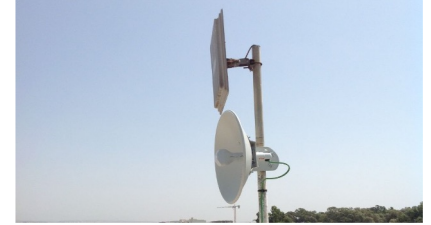
Point to Point Wifi: 2-way, (requires line of sight)
